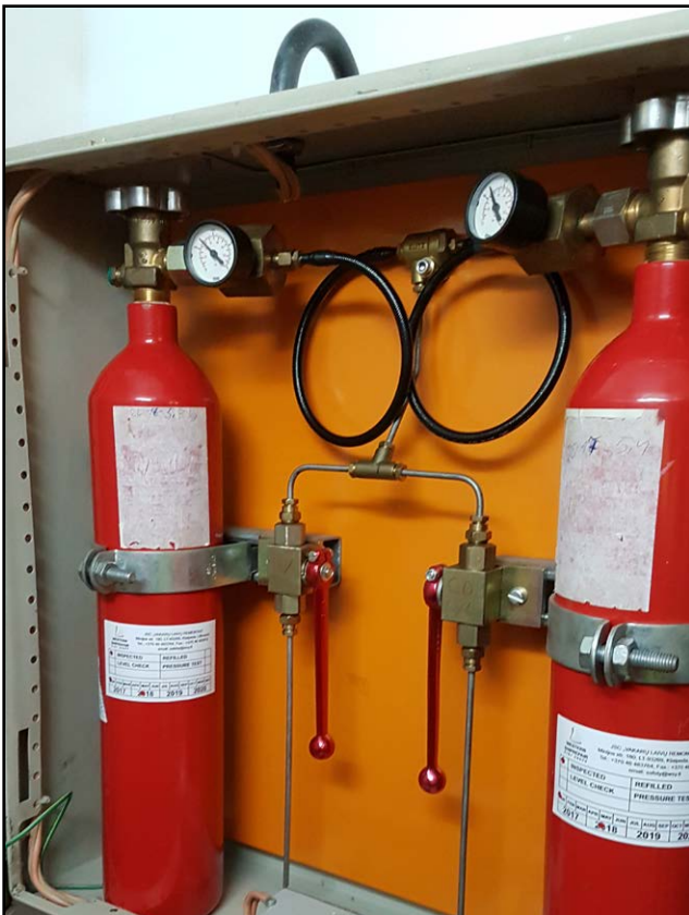
Figure 10: CO 2 remote release station
