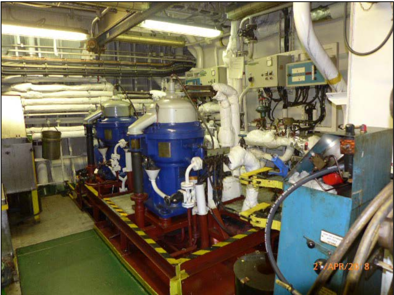
Figure 2: Engine room purifier room
