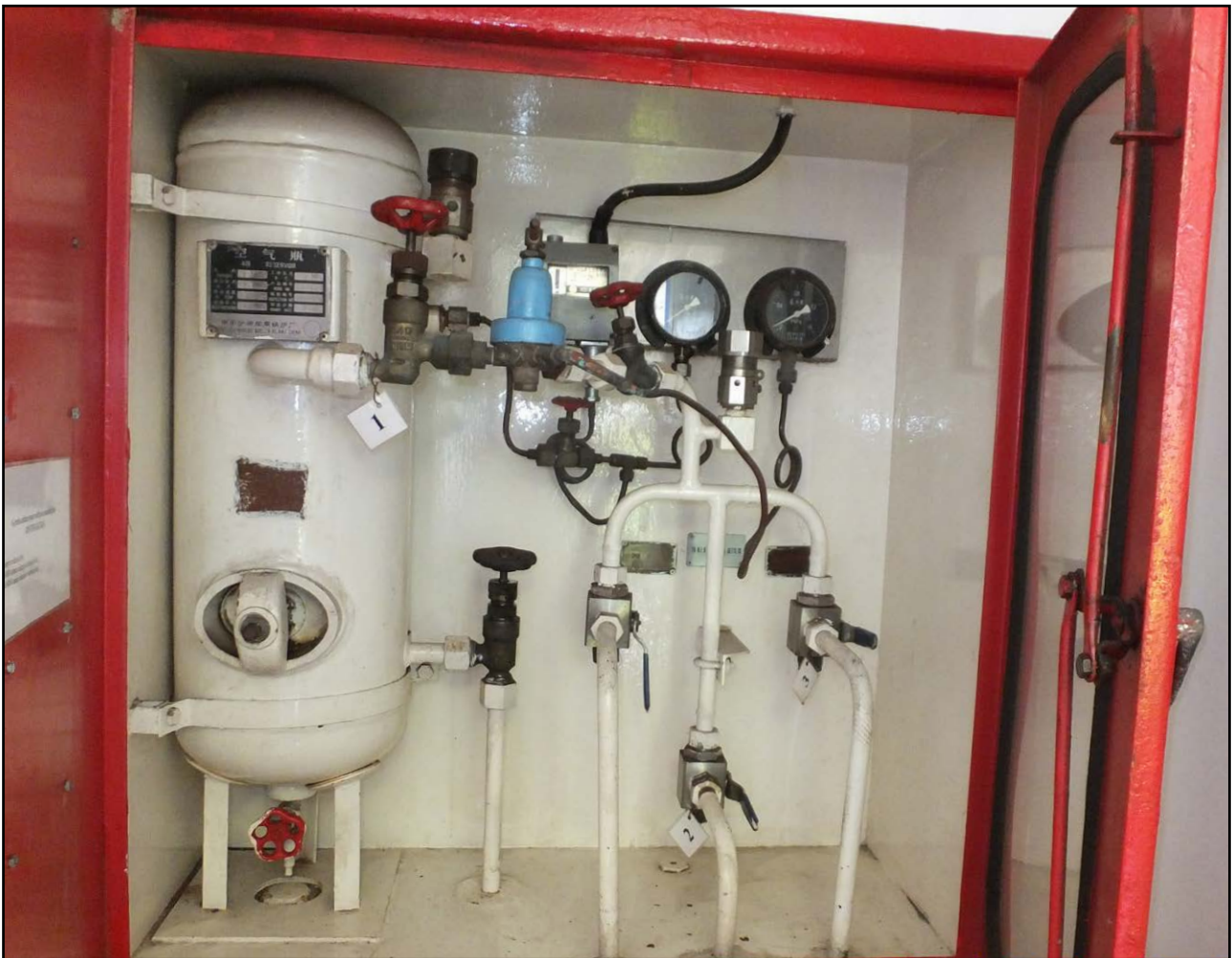
Figure 5: Control station for the engine room fuel systems' quick-closing valves
