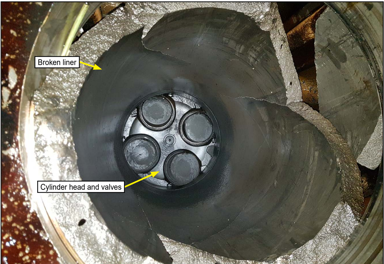
Figure 22: B5 liner (looking up to inlet/exhaust valves from engine sump)
