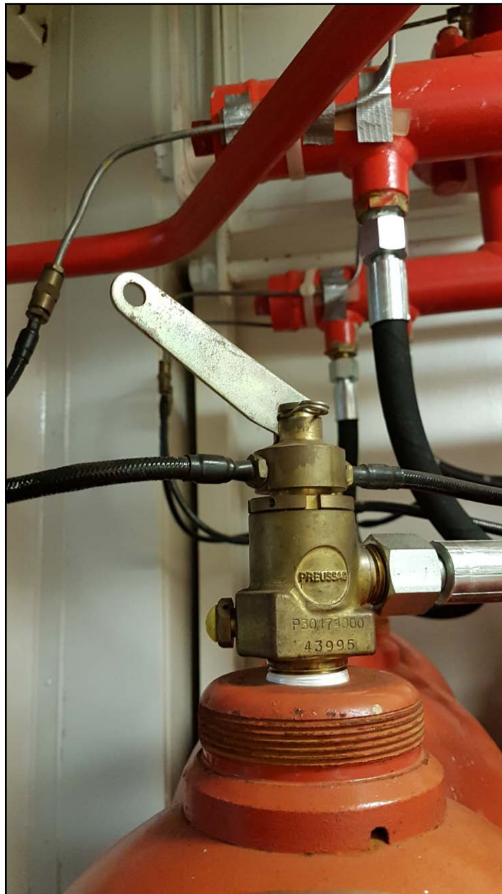
Figure 28: Carbon dioxide bottle operating valve
