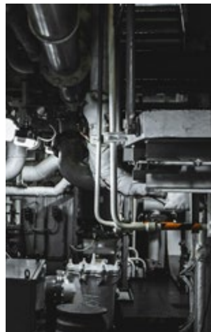
Figures 2 and 3 show a sample line found blocked when no flow observed from 15ppm bilge alarm outlet.
