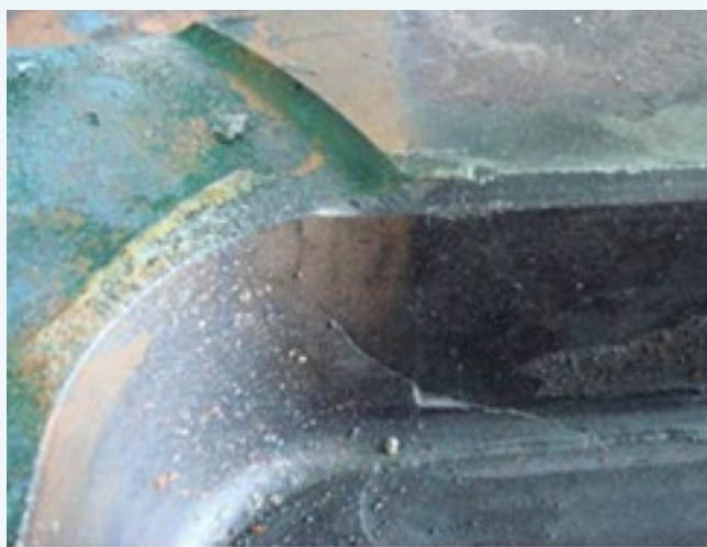
(a) Fatigue crack initiation
