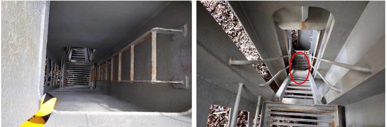
Figure 2: Cargo Hold No. 1 aft access ladder. The vertical ladder leading from the booby hatch to the upper platform is shown in the photograph on the left. The inclined ladder between the upper and intermediate platforms is shown in the photograph on the right. The location where the C/E, ETO, and Fitter were found at the bottom of the ladder and on the intermediate platform is circled in red. The cargo of scrap metal is visible in both photographs.
