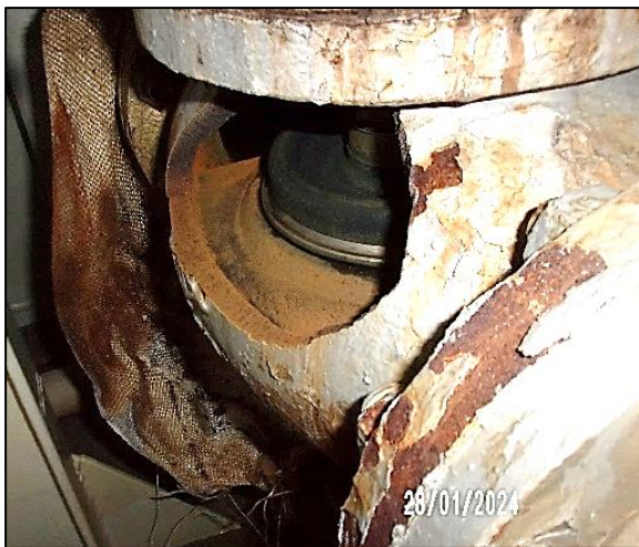
Figure 2: Ruptured steam inlet valve
