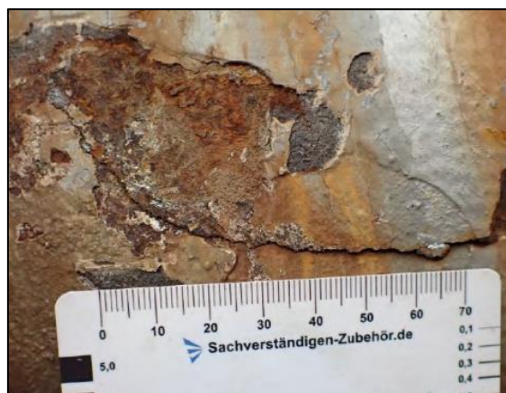
Figure 8: Close up of crack
