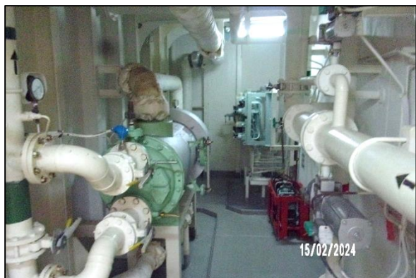
Figure 3: View of heater when entering
