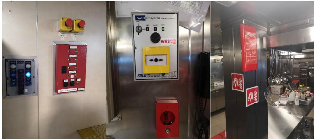
Galley firefighting systems and emergency stops
