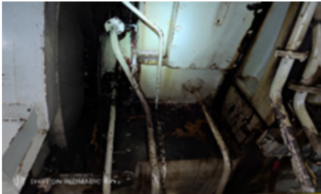
Figure 15.1 Oil leaks in engine room
