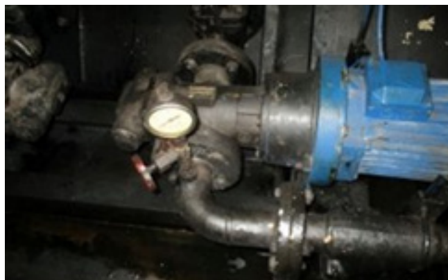
Figure 16.2 Oil leaks in engine room
