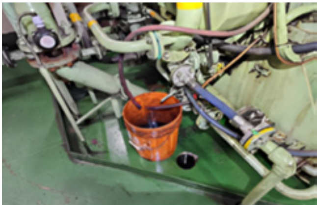
Figure 16.1 Oil leaks in engine room
