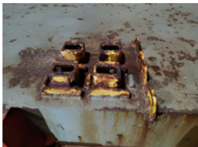
Figure 1 Corroded container securing points
