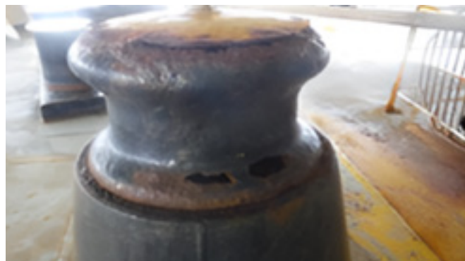
Figure 14 Fairlead in poor condition
