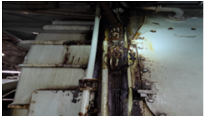
Figure 15.2 Oil leaks in engine room
