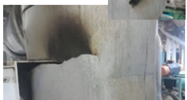
Figure 18 Signs of exhaust leak
