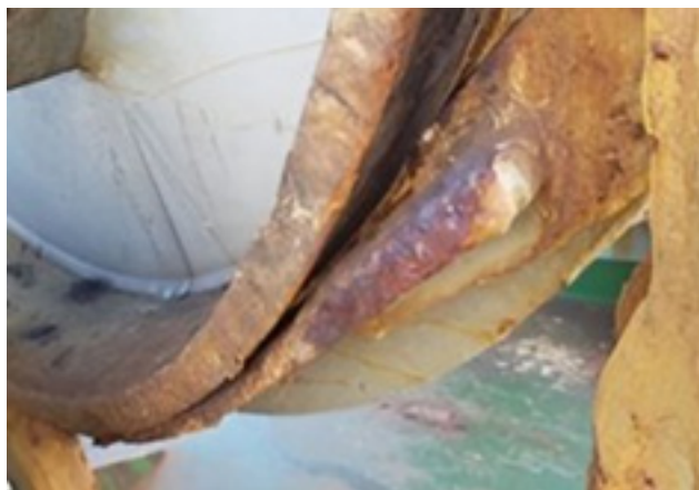
Figure 12 Worn brake lining
