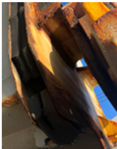
Figure 20 Gaps in rubber packing
