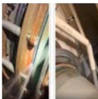
Figure 1: Sea water discharging through seal face
