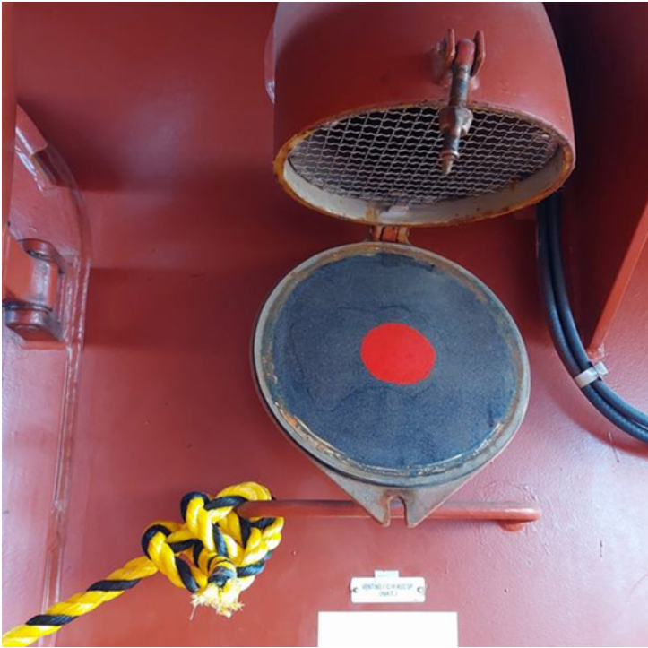
Figure 4: Ventilation of the CH No. 1 Access Space.
